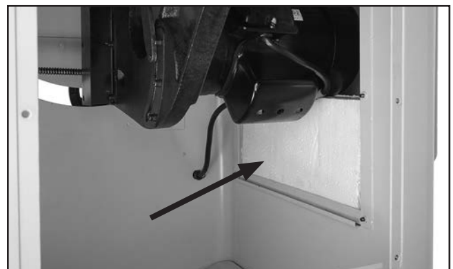
Figure 29. Location of styrofoam block to be removed.
